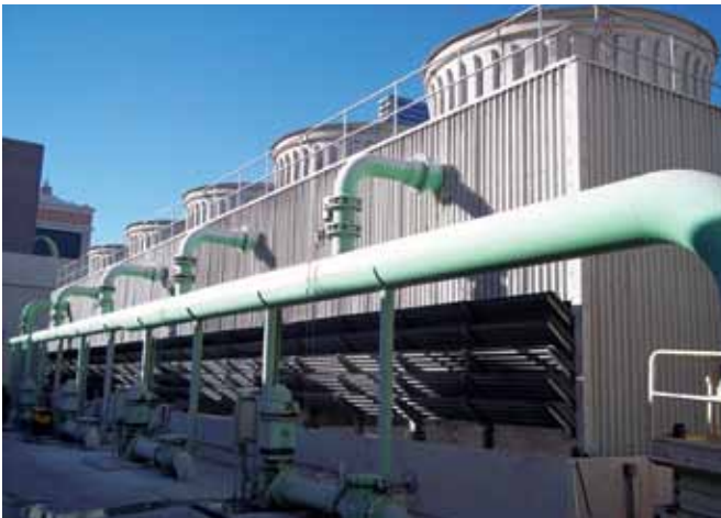
Cooling towers may be overemphasized as a means of Legionella transmission
